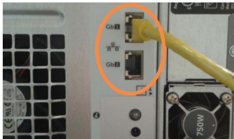
Figure 16-5: Ethernet ports used for LIS connectivity
